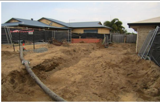
450mm sewer suspected partial collapse
