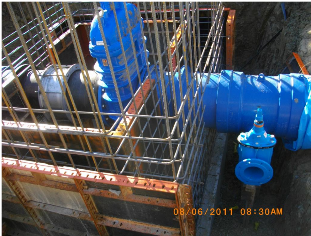
South Mackay Trunk Main - Valve Pit under construction, one of many along the pipeline
