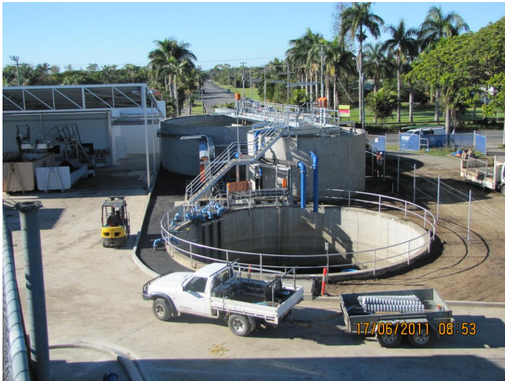
Nebo Road WTP - New Sludge Dewatering Circuit operating in treatment process
